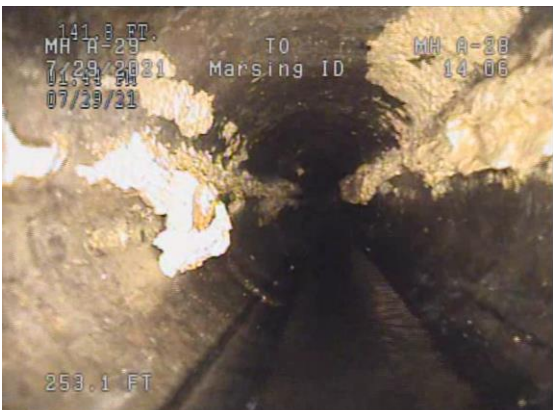
Picture of grease buildup in city sewer main on 3 rd round of cleaning.
